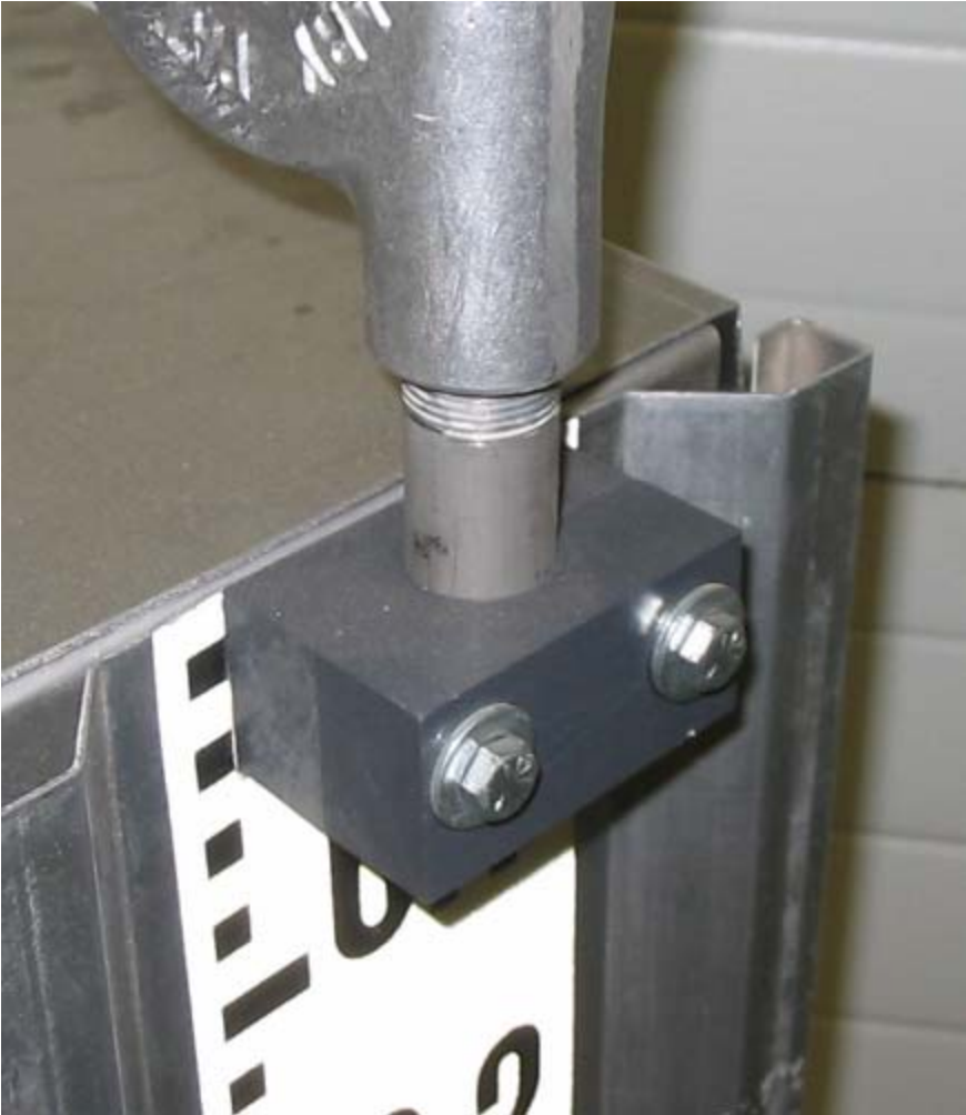
CABLE GUIDE FITTED INTO PVC SUPPORT AT TOP OF GAUGE BOARD
